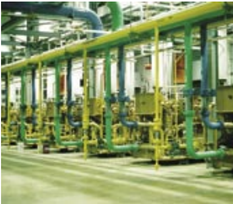
Stand-by Generation Facility
